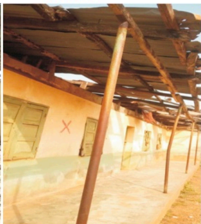
Dilapidated Classroom at St. Thomas's Catholic Nursery & Primary School, Odo-Oro
